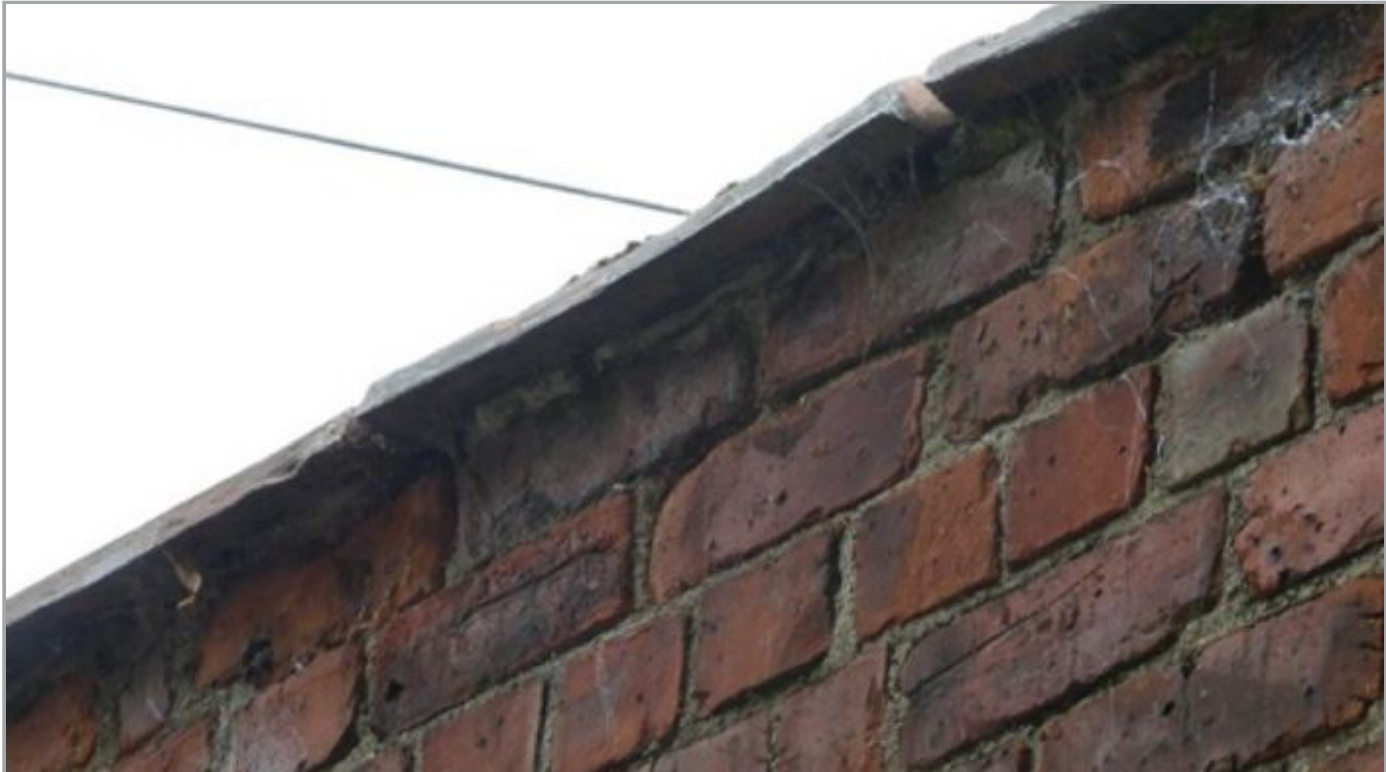
Solid Construction Eroding Pointing
