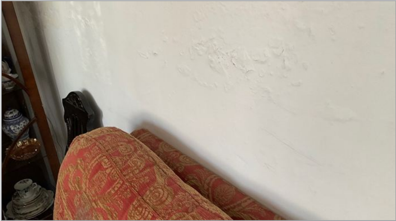
Damp Patches/Salt Staining
