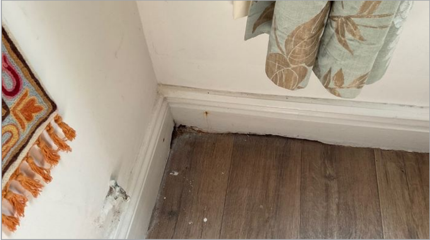
Damp Patches/Salt Staining
