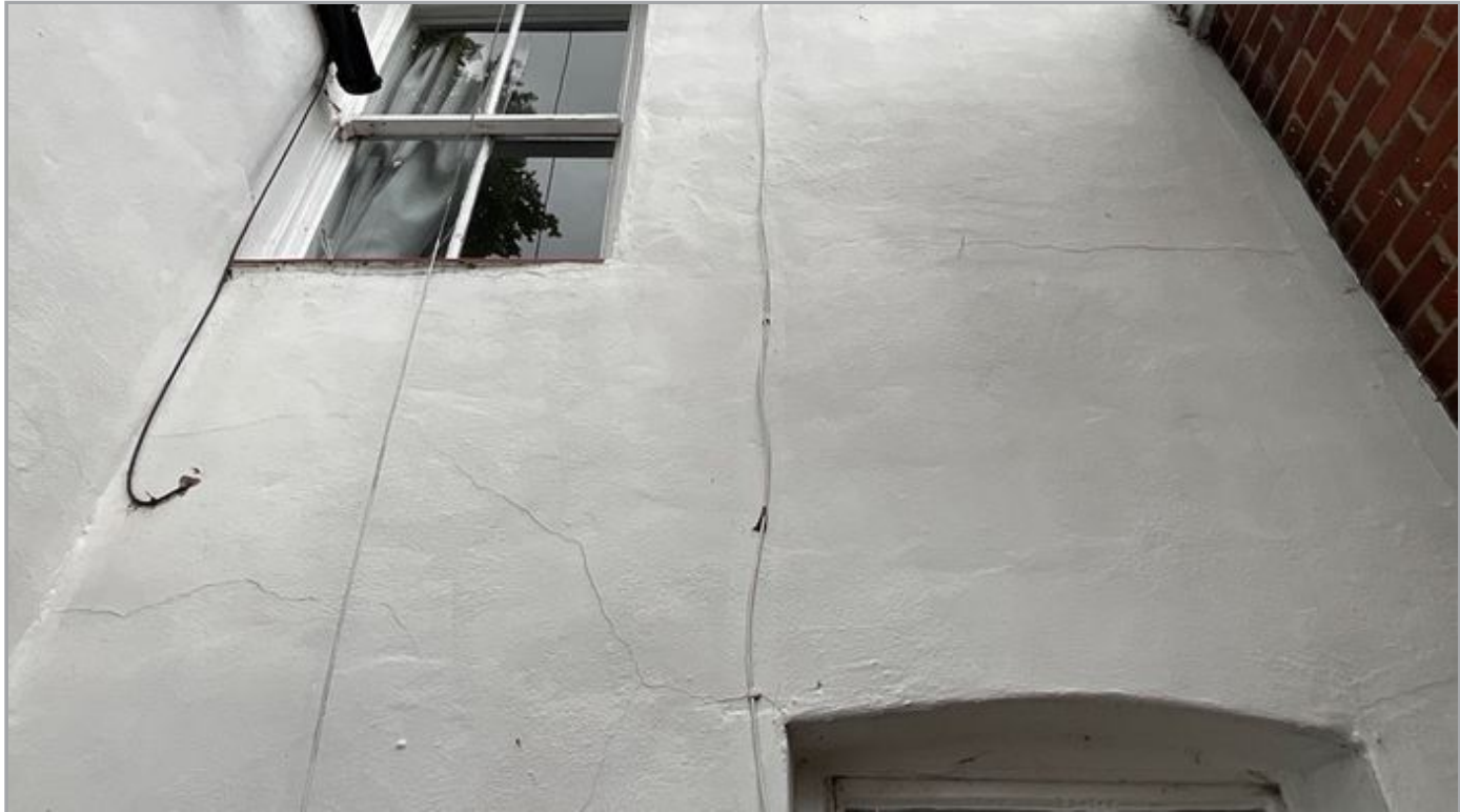
Render Cracking/Thermal Movement
