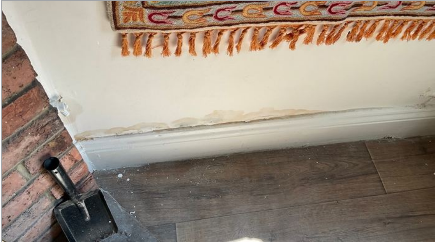
Damp Patches/Salt Staining
