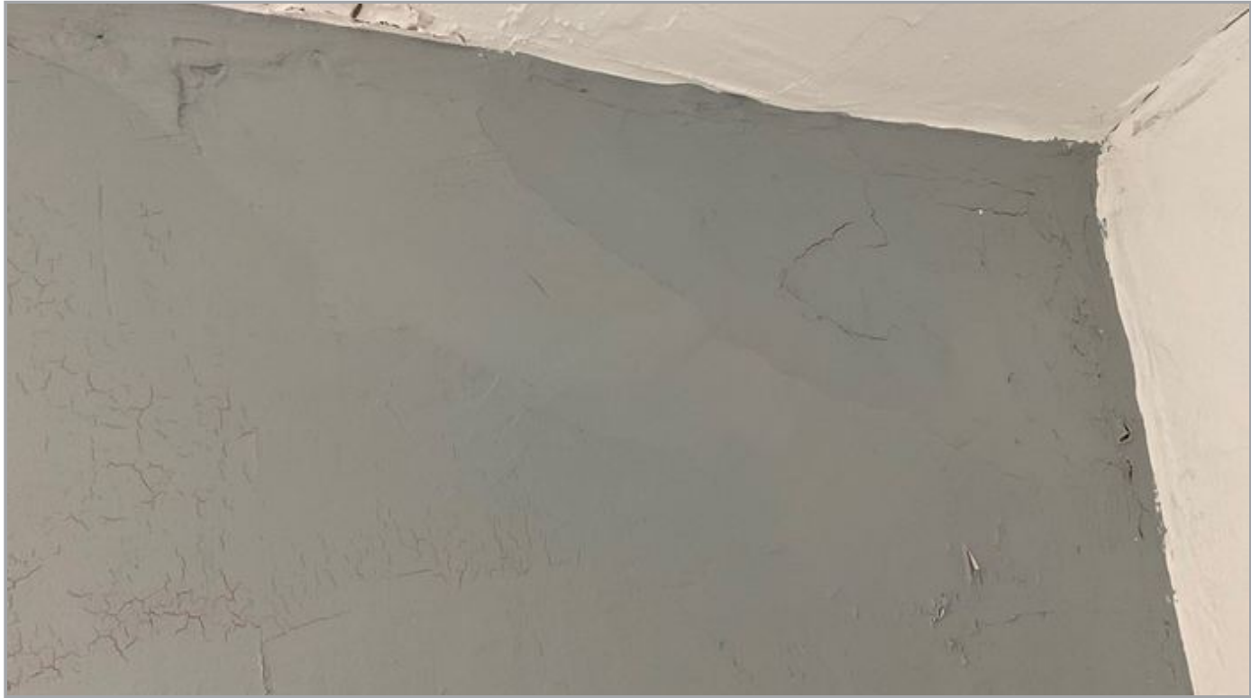
Damp Patches/Salt Staining Bathroom
