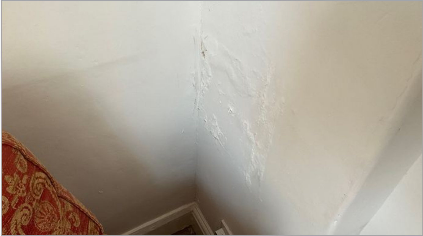
Damp Patches/Salt Staining
