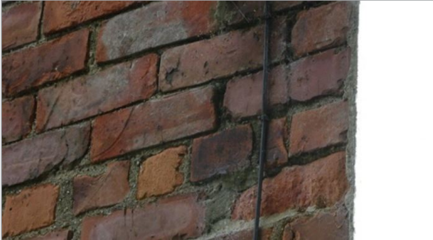
Solid Construction Eroding Pointing
