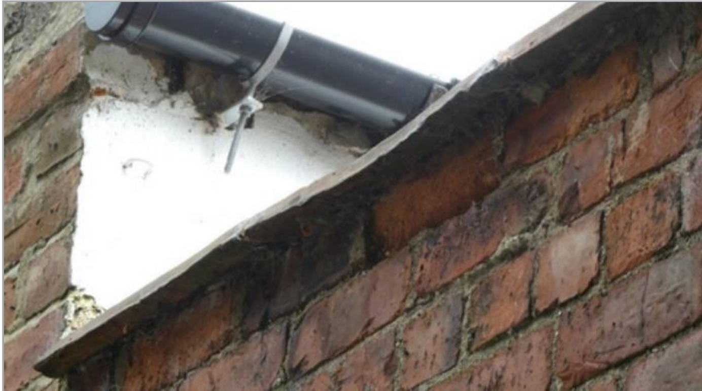
Solid Construction Eroding Pointing
