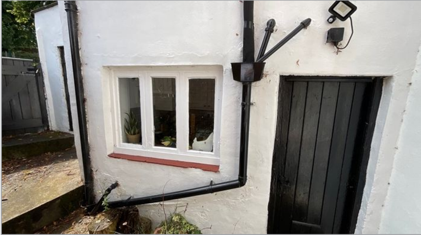
Misconnection/Overloading Drainage Pipework
