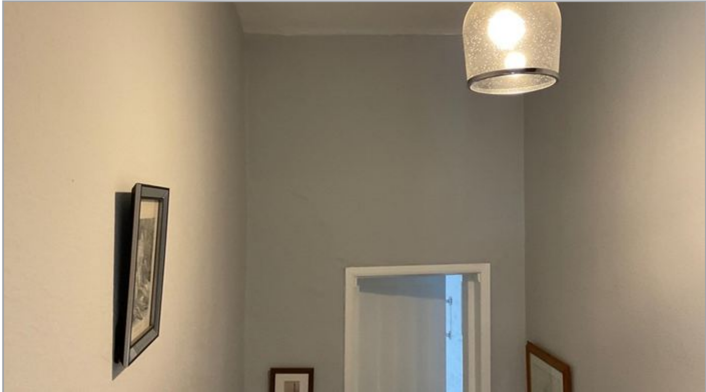
Possible Ongoing Structural Movement
