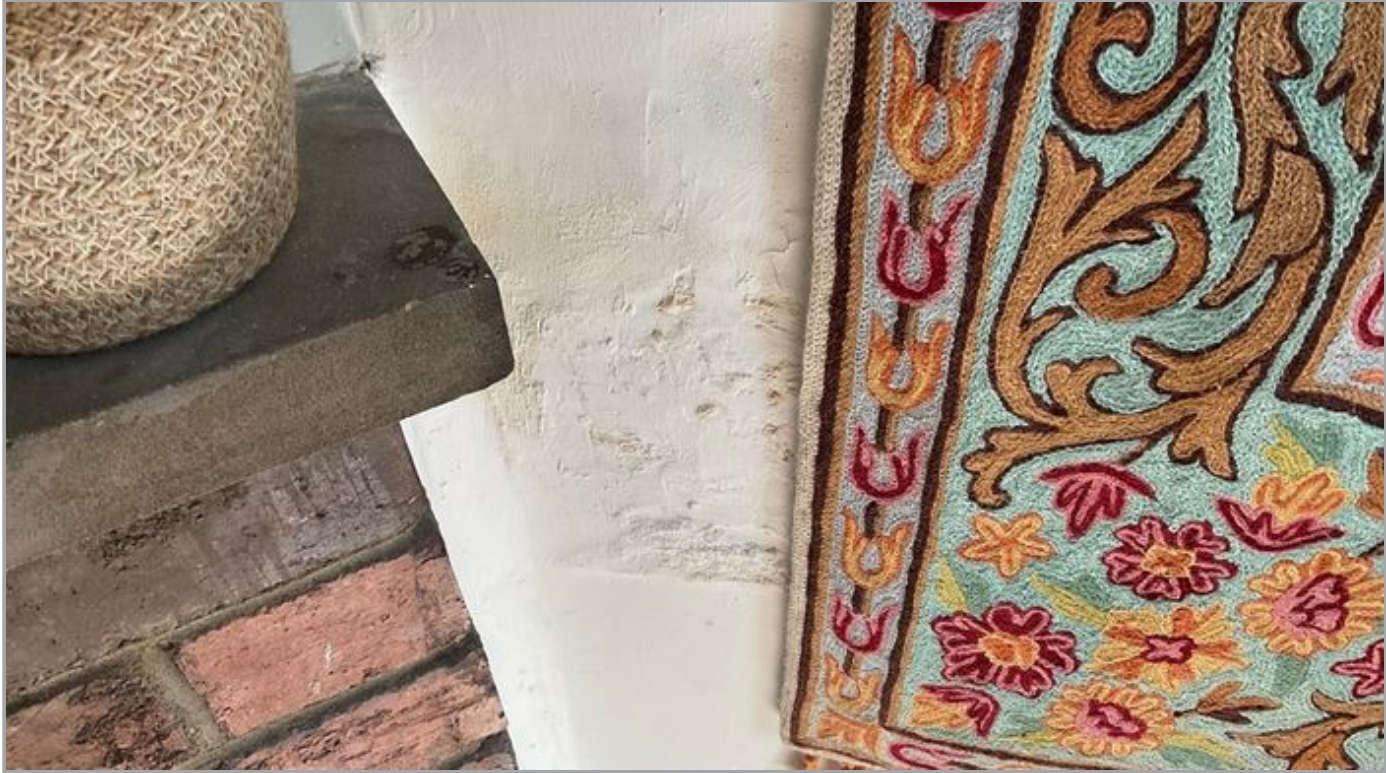
Damp Patches/Salt Staining
