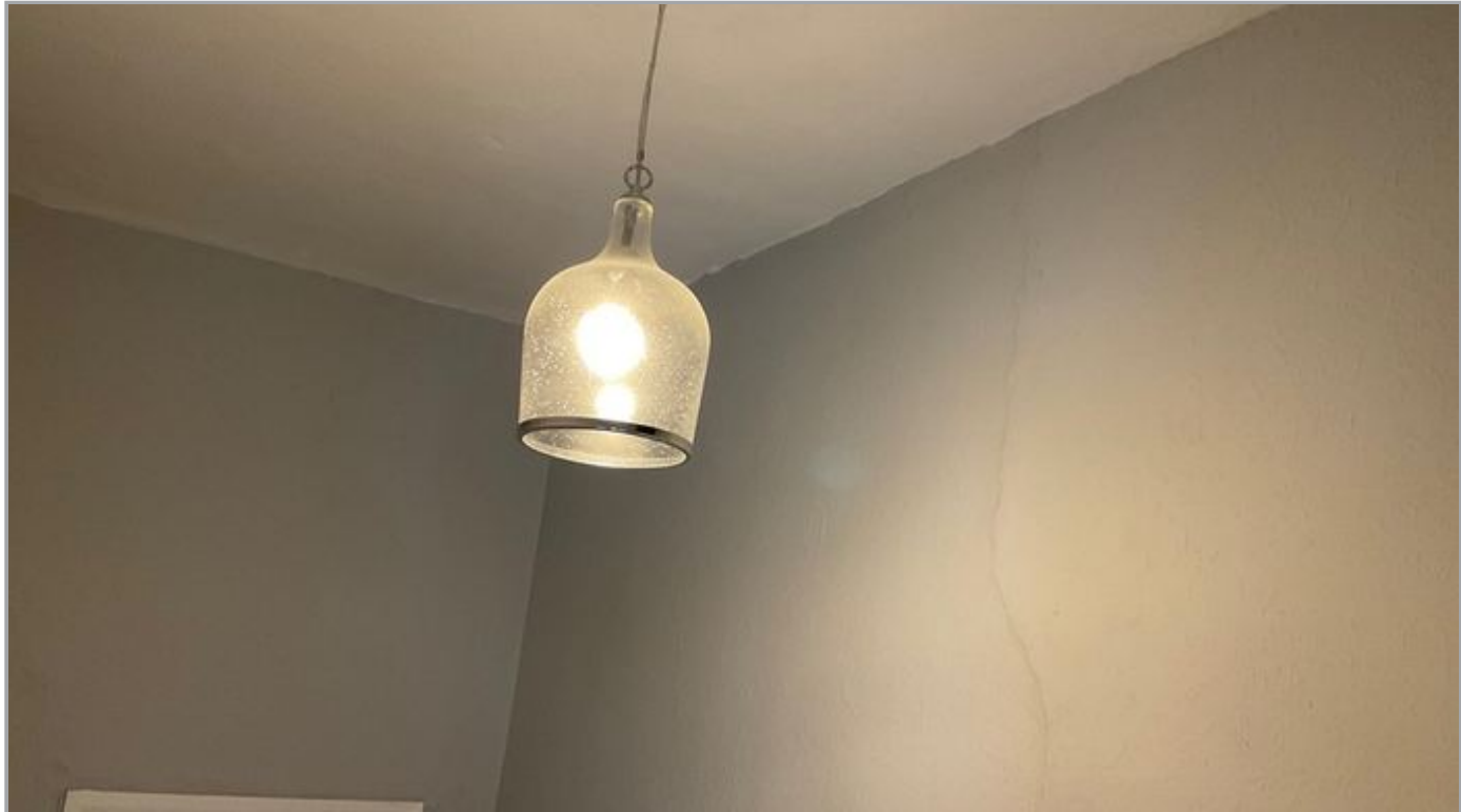
Possible Ongoing Structural Movement
