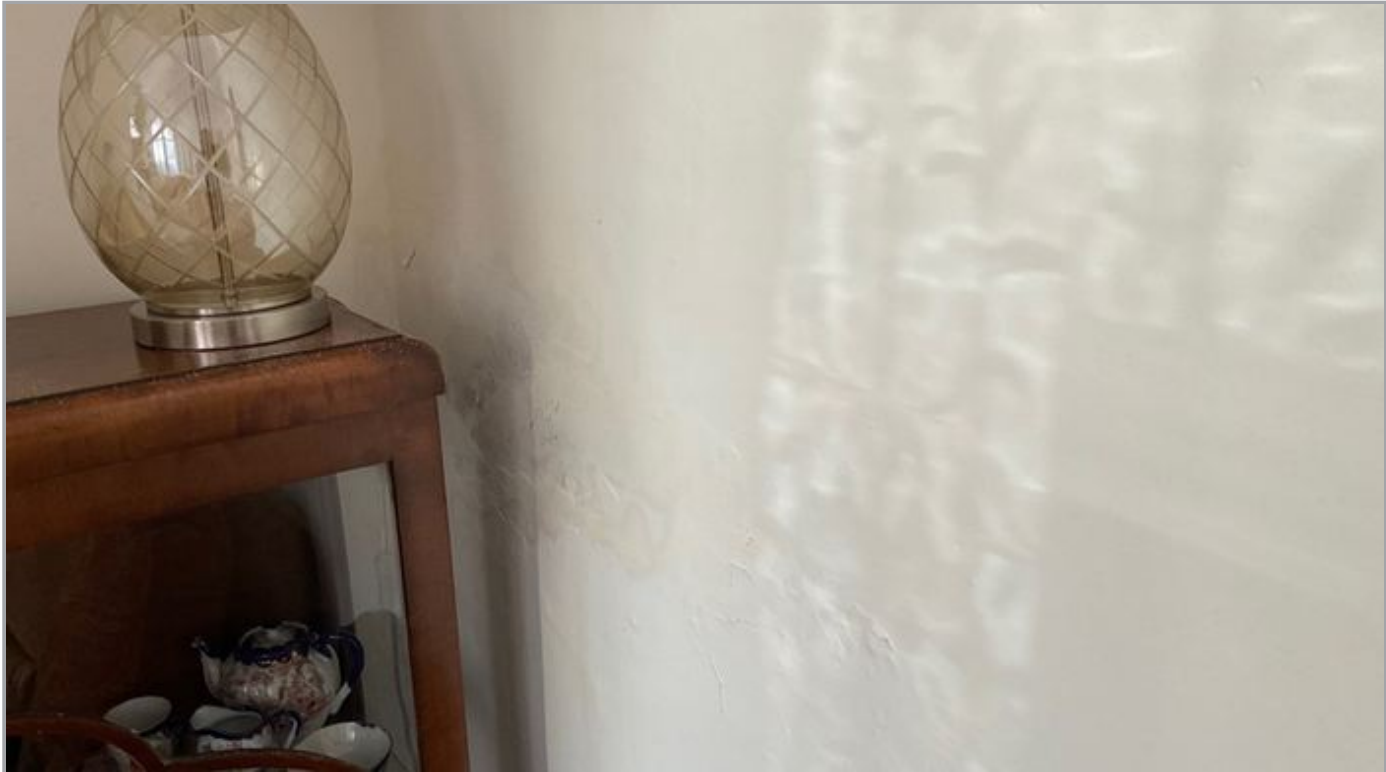
Damp Patches/Salt Staining
