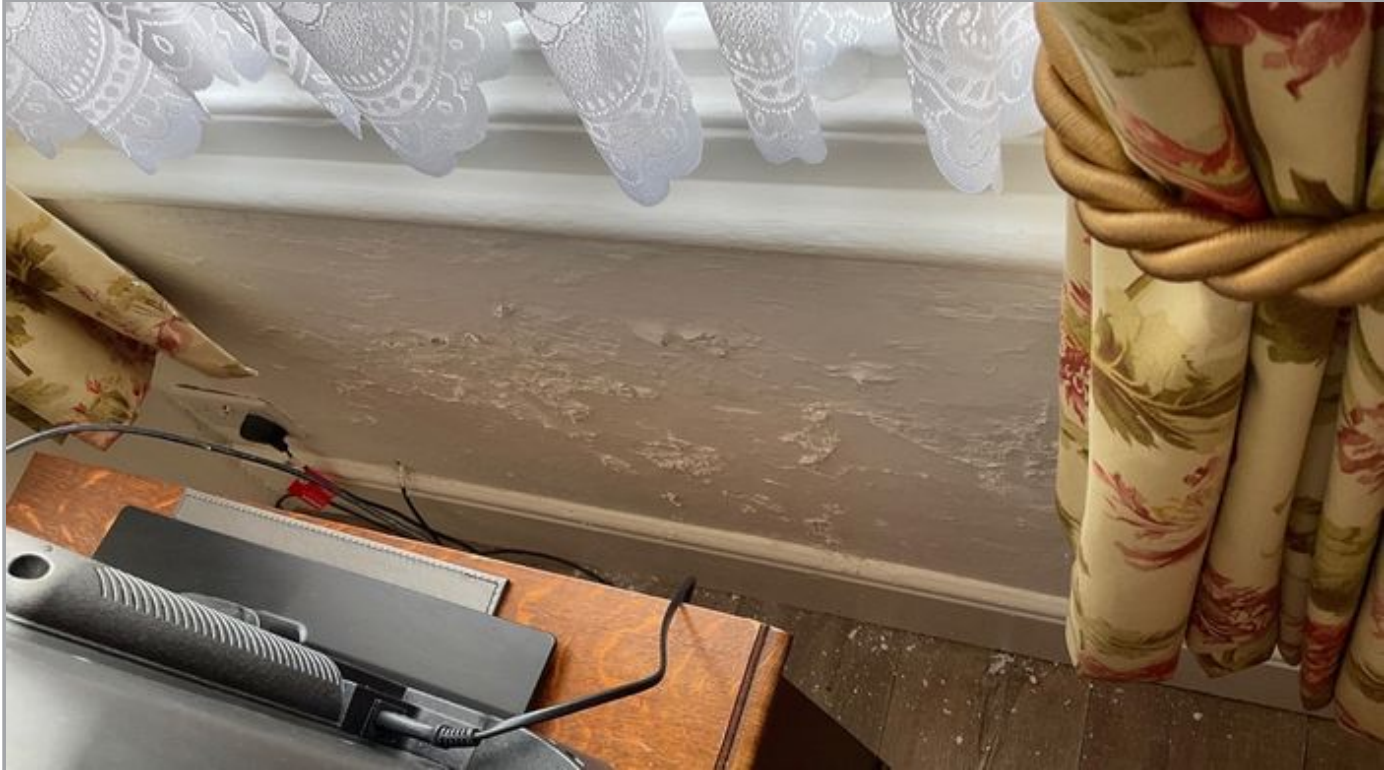
Damp Patches/Salt Staining
