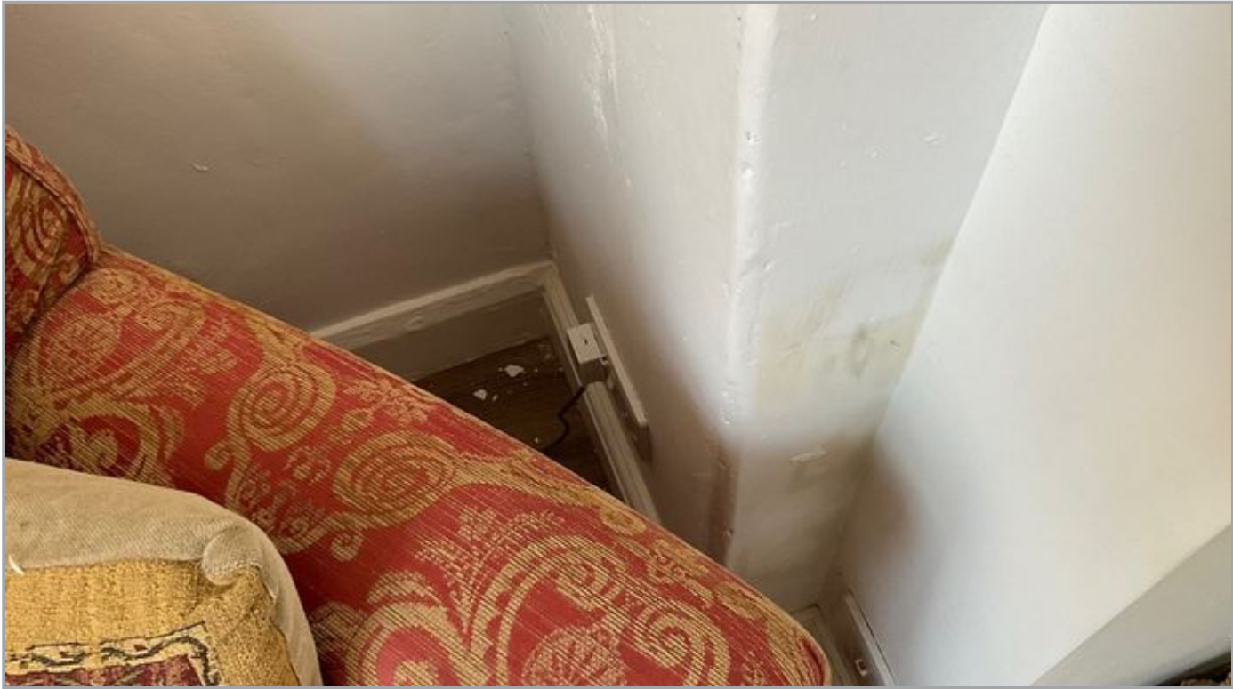
Damp Patches/Salt Staining
