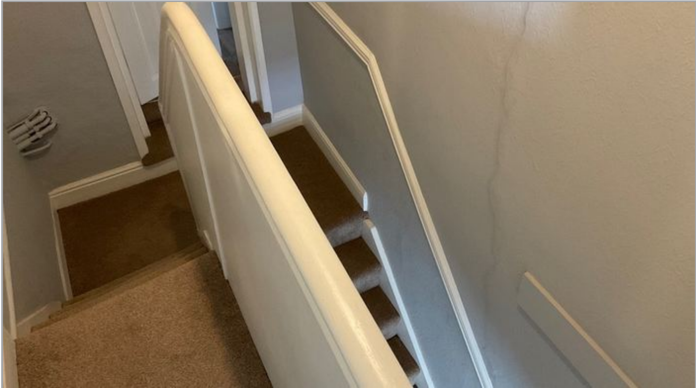
Possible Ongoing Structural Movement
