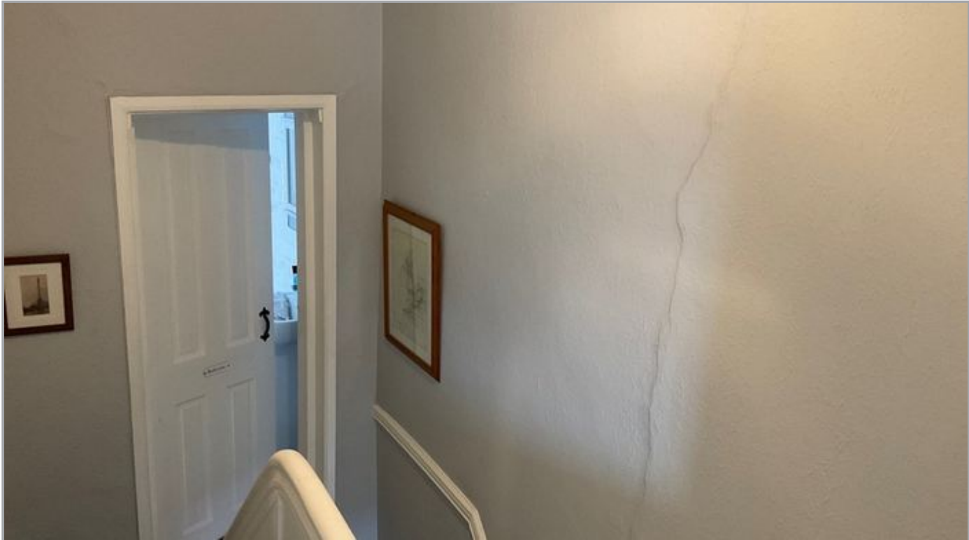
Possible Ongoing Structural Movement
