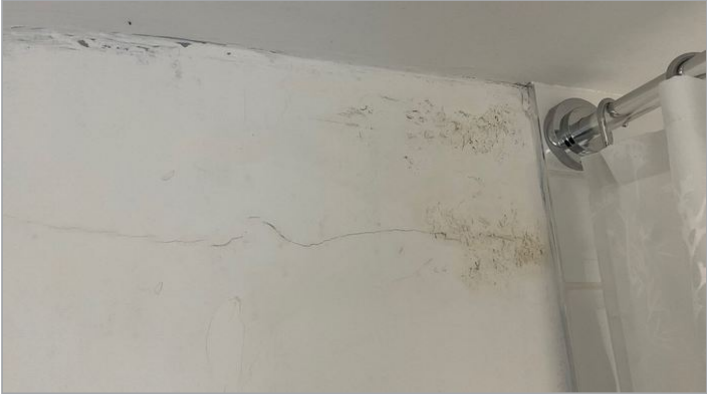
Damp Patches/Salt Staining Bathroom
