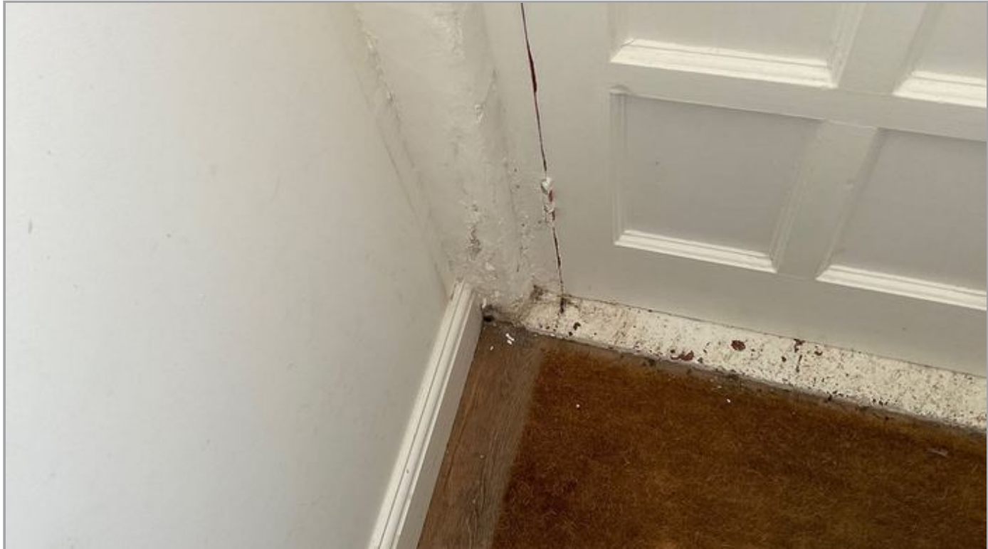
Damp Patches/Salt Staining
