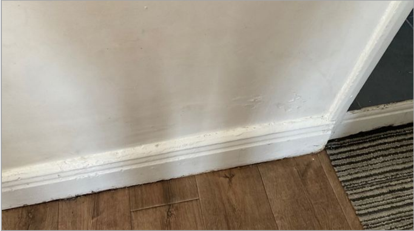
Damp Patches/Salt Staining
