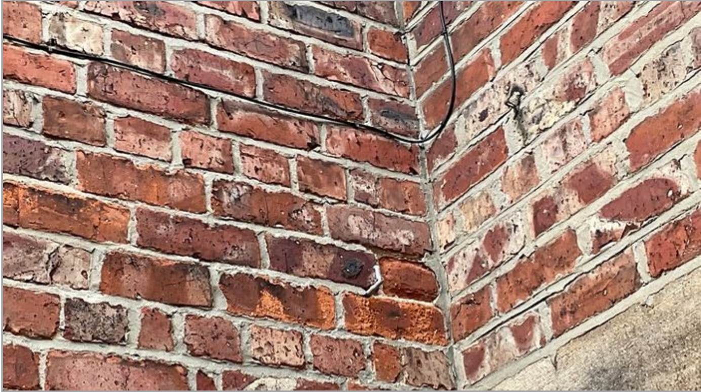
Solid Construction Eroding Pointing
