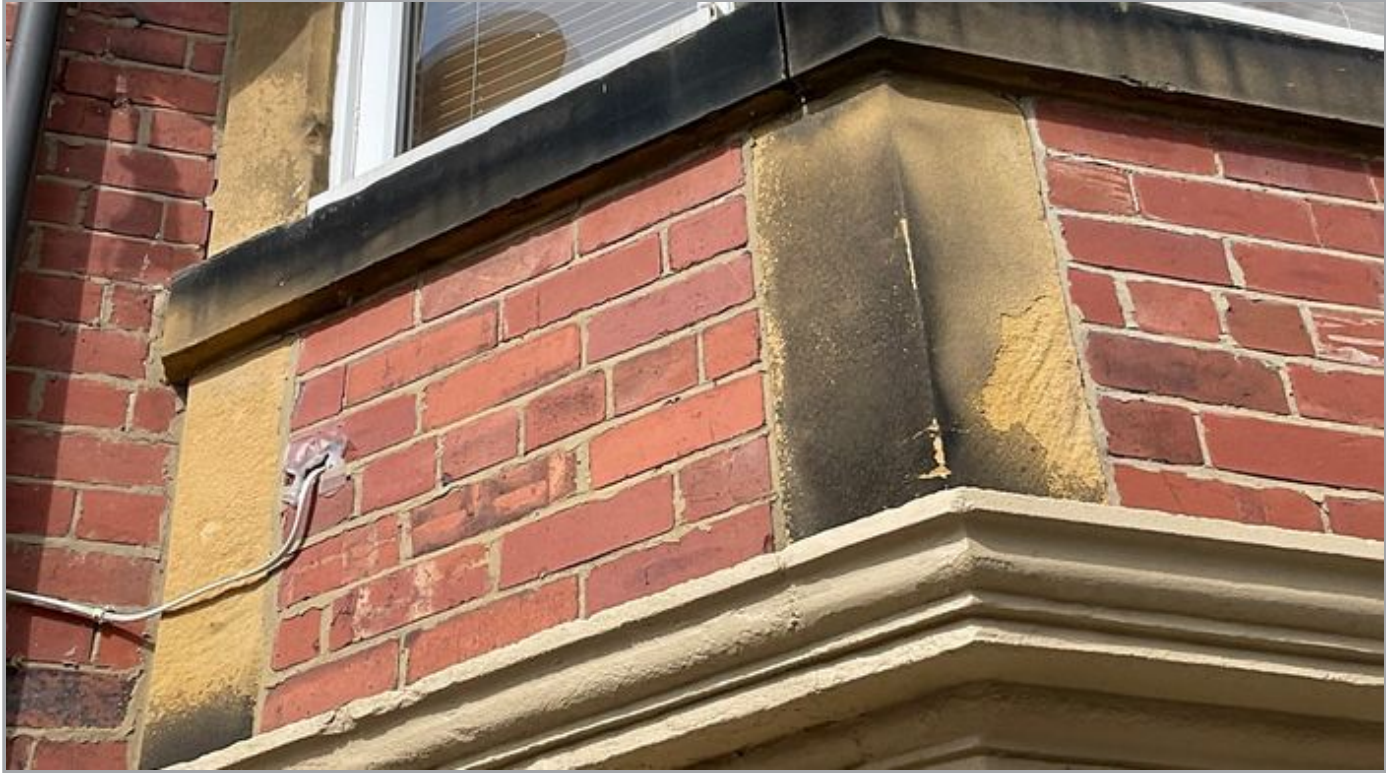
Solid Construction Eroding Pointing
