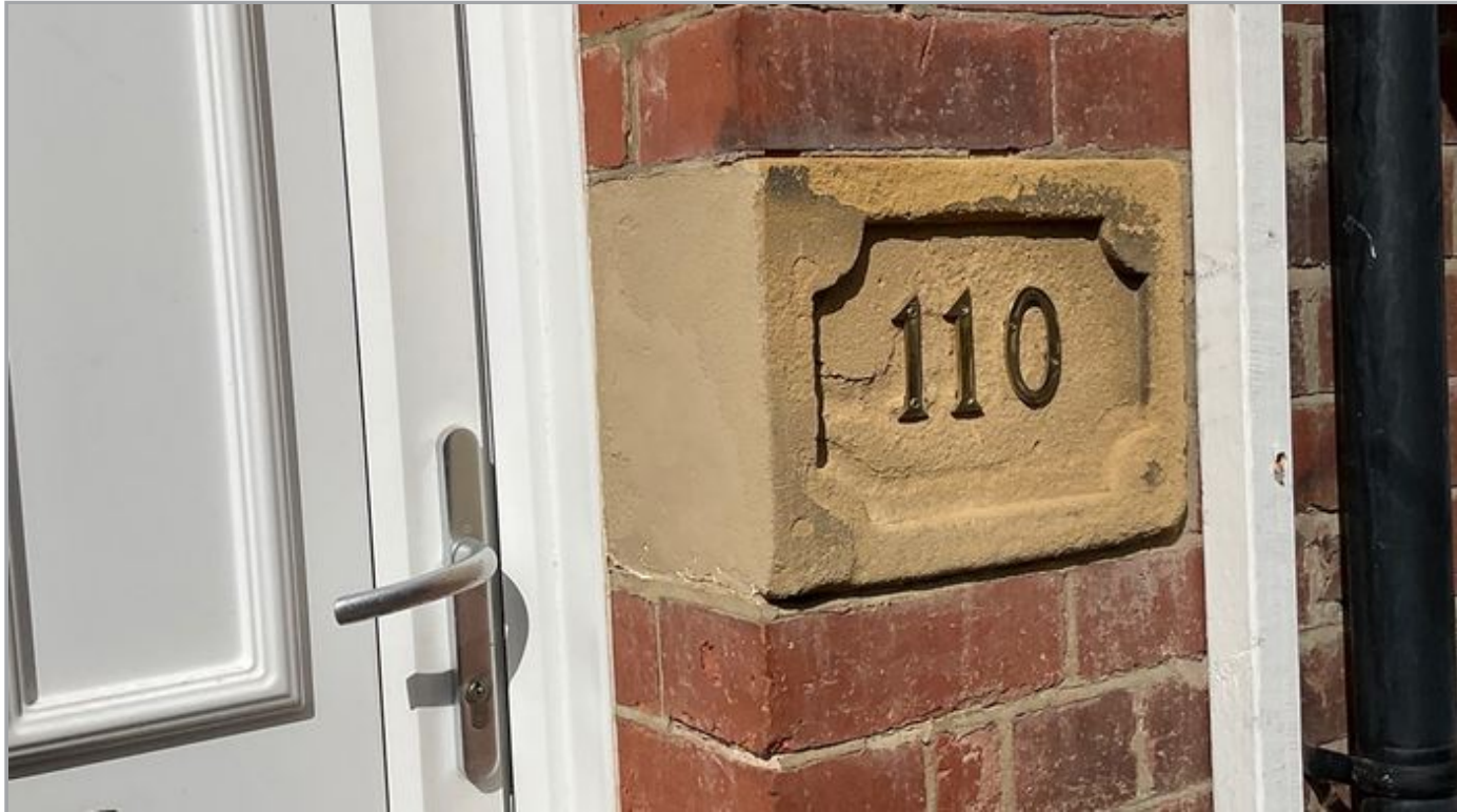
Solid Construction Eroding Pointing
