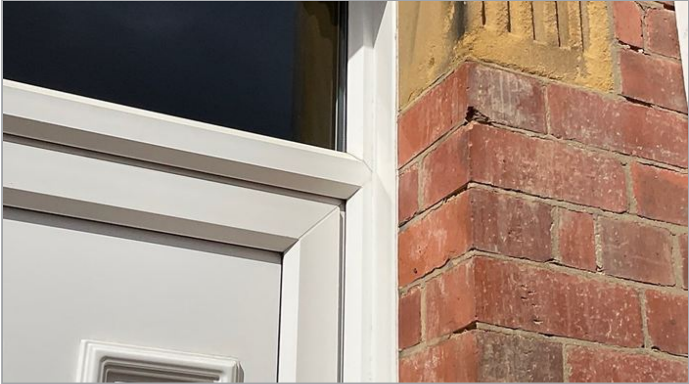
Solid Construction Eroding Pointing
