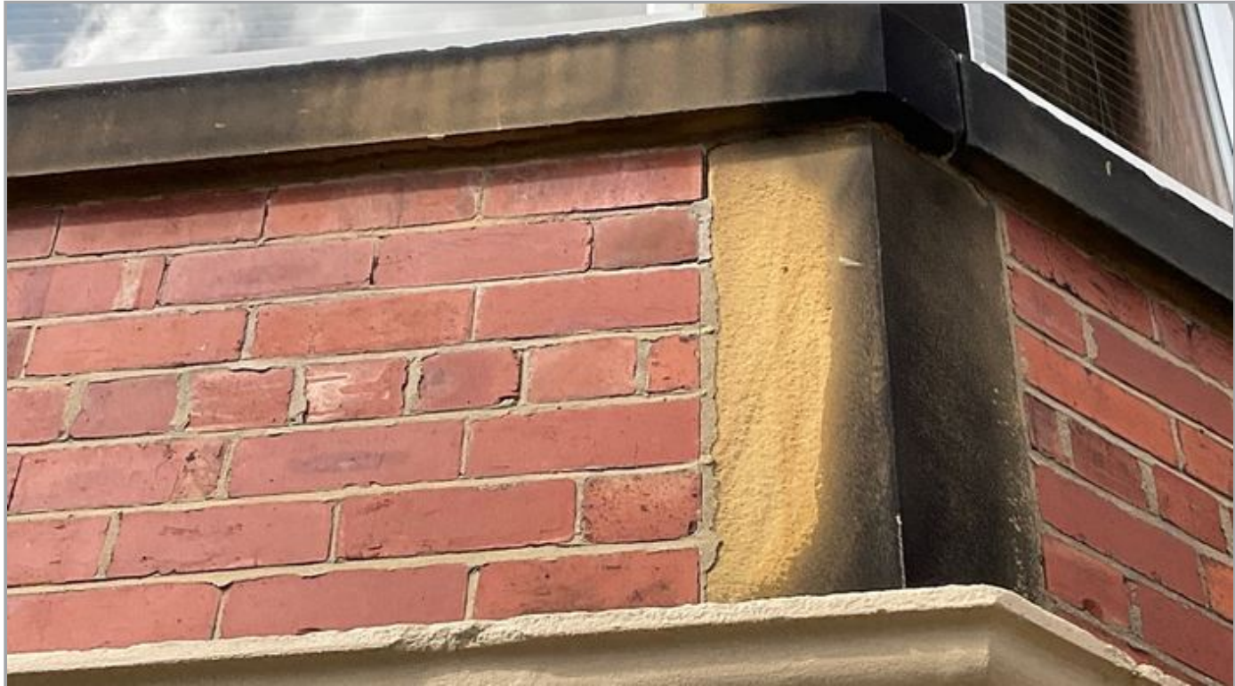
Solid Construction Eroding Pointing
