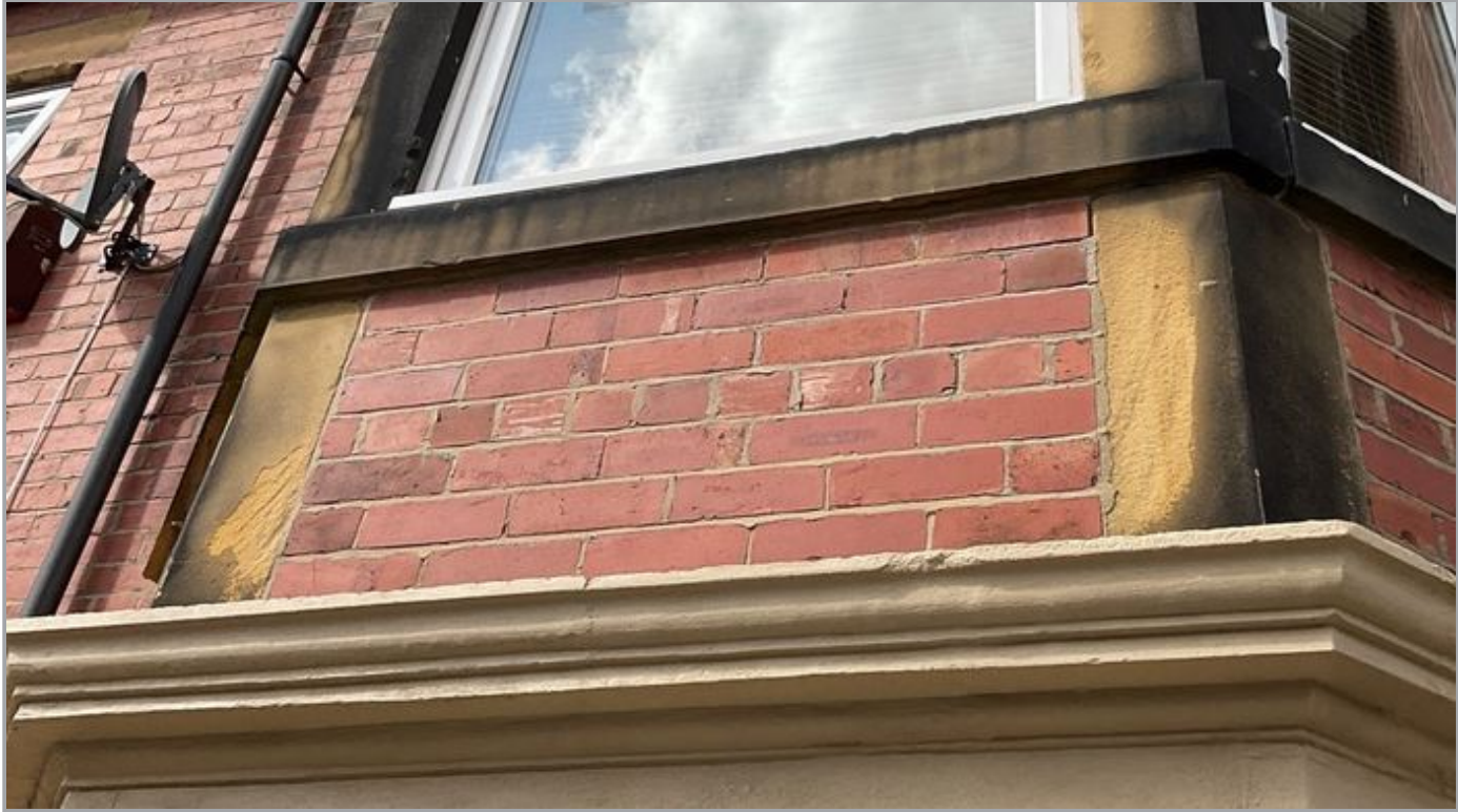
Solid Construction Eroding Pointing
