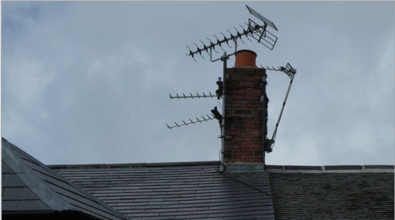
Stack Leaning Ongoing Monitoring
